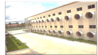
Evaporative Cooling Pad system
