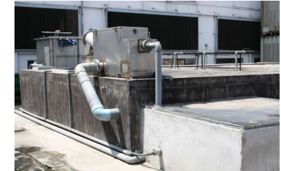
Wasted water treatment system
