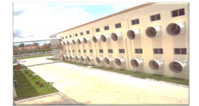
Evaporative Cooling Pad system
