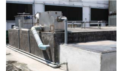
Wasted water treatment system
