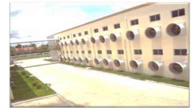
Evaporative Cooling Pad system
