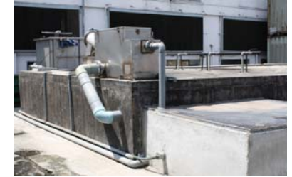
Wasted water treatment system
