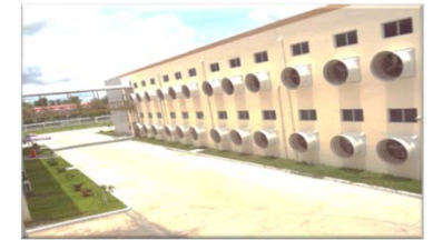
Evaporative Cooling Pad system
