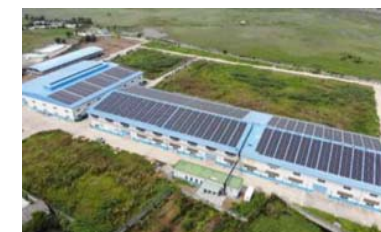
Solar panel on rooftop
