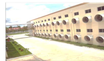
Evaporative Cooling Pad system
