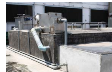
Wasted water treatment system
