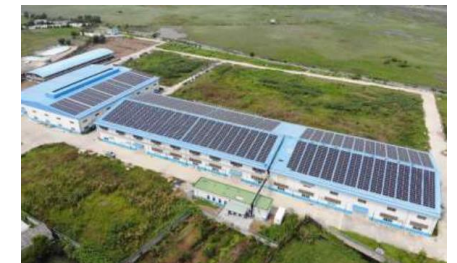
Solar panel on rooftop
