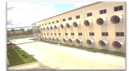
Evaporative Cooling Pad system
