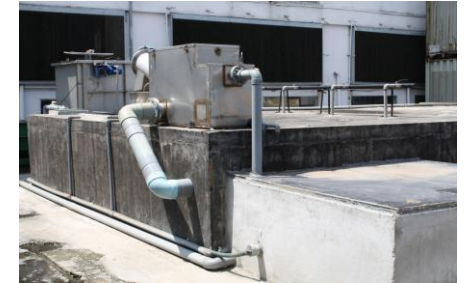
Wasted water treatment system
